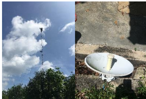
Gambar 33. Pengecekan radio Power Beam
